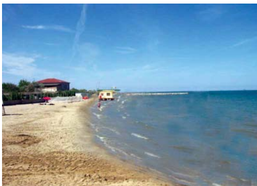
Figure 3. Northern beach: erosion.
