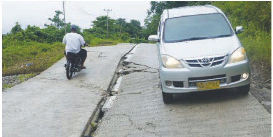
Figure 3: Slumping in tropical roads (photo © Mohammed Alamgir)
